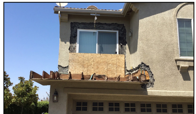
Balcony Dryrot Damage, Building 8
